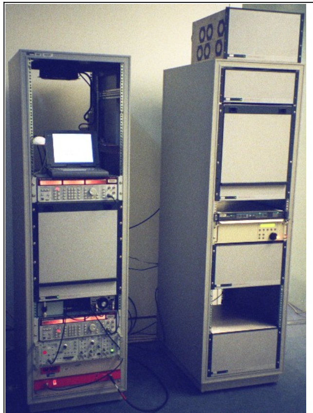
Picture 2 - Transmission Equipment Racks
